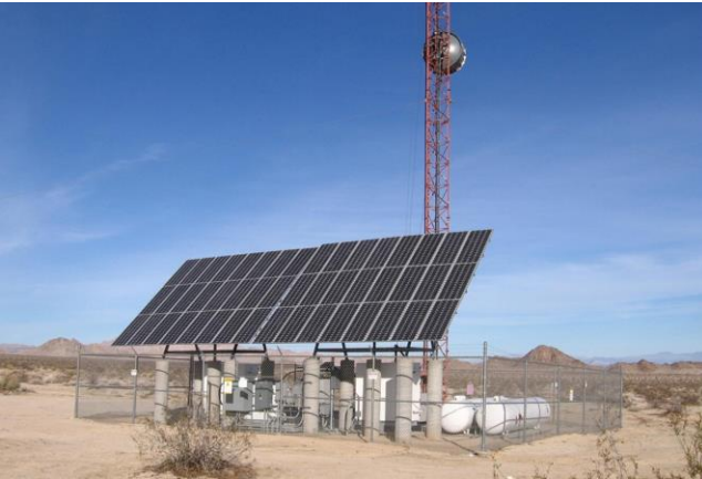
Off-Grid Power Source replacing diesel power with solar+storage
